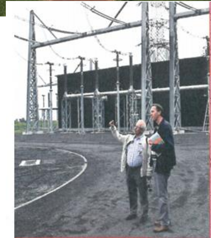
Goffinet and STRI's Igor Gutman examine insulator strings on towers entering Horta Substation.
